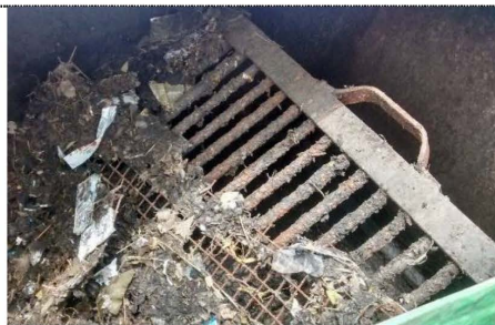
Screen inside feed tank
